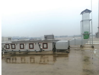
Tail gas treatment devices at laboratories in Beijing plant
