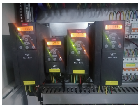
Variable frequency control system
