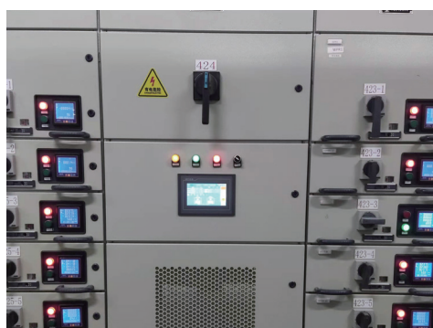
Active power filter
