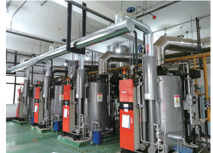
Low-nitrogen burners used for the gas-fired boilers in Beijing plant
