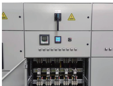
Reactive compensation technology for power grid system
